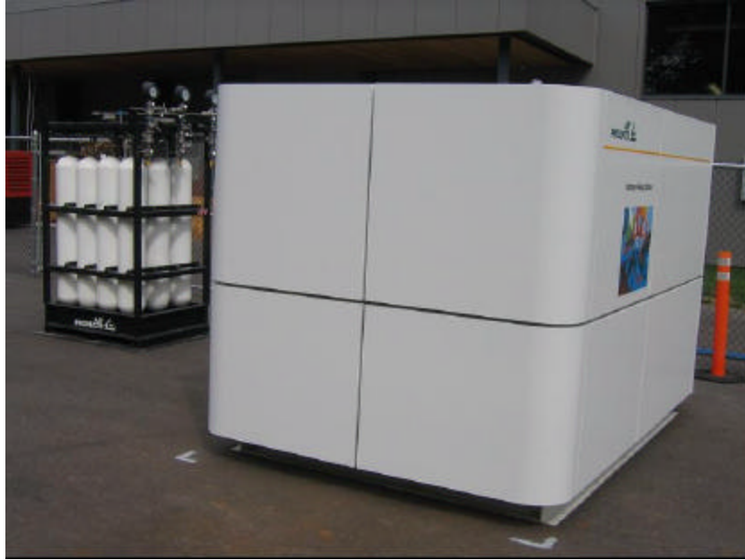
Figure 1: Air Products storage (left) and compression (right) modules for the EVERmont project
